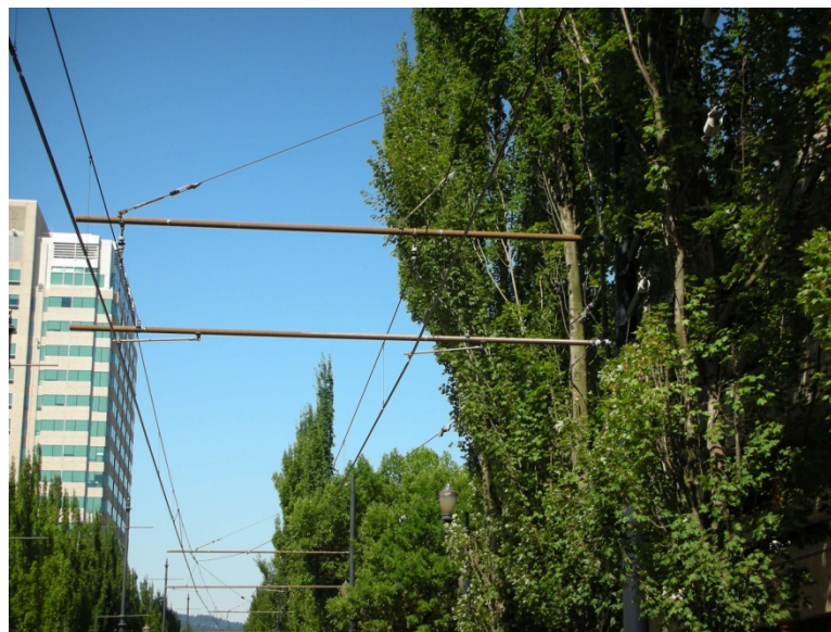
Fig. 6 - Typical Simple Catenary Cantilever
