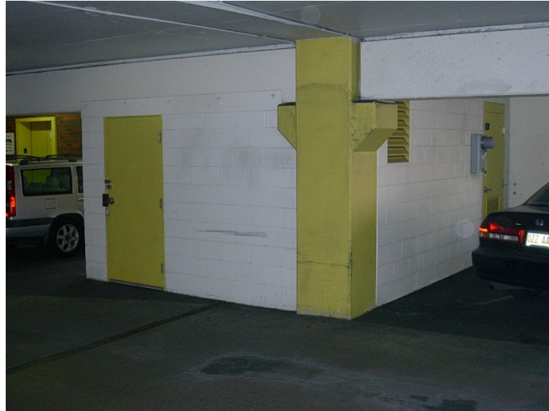
Fig. 5 – Parking Garage Enclosure for Low Power Substation
